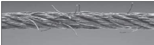
Cable with Corrosion
